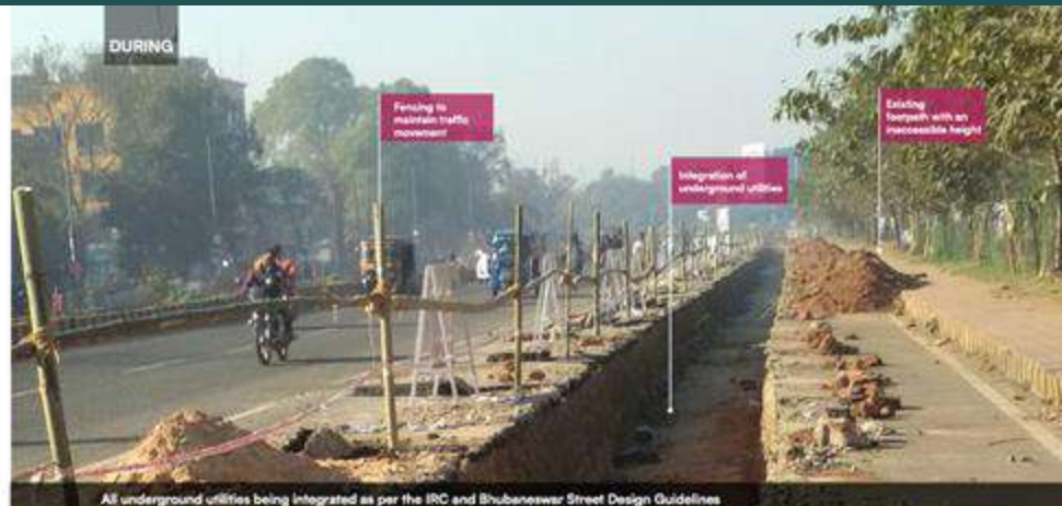
All underground utilities being integrated as per the IRC and Bhubaneswar Street Design Guidelines
